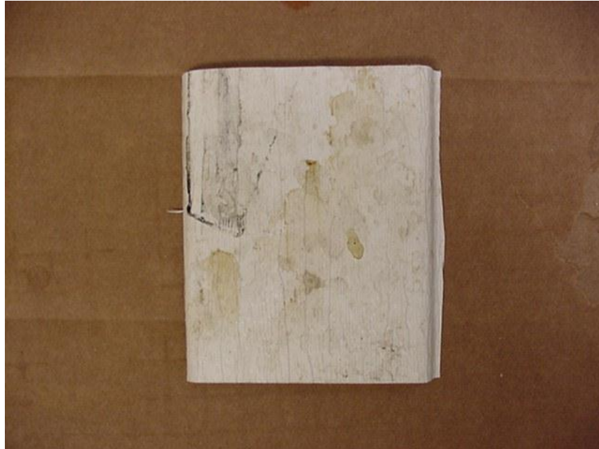
Figure 6: A siding sample with mold and stain, before CMSR.
